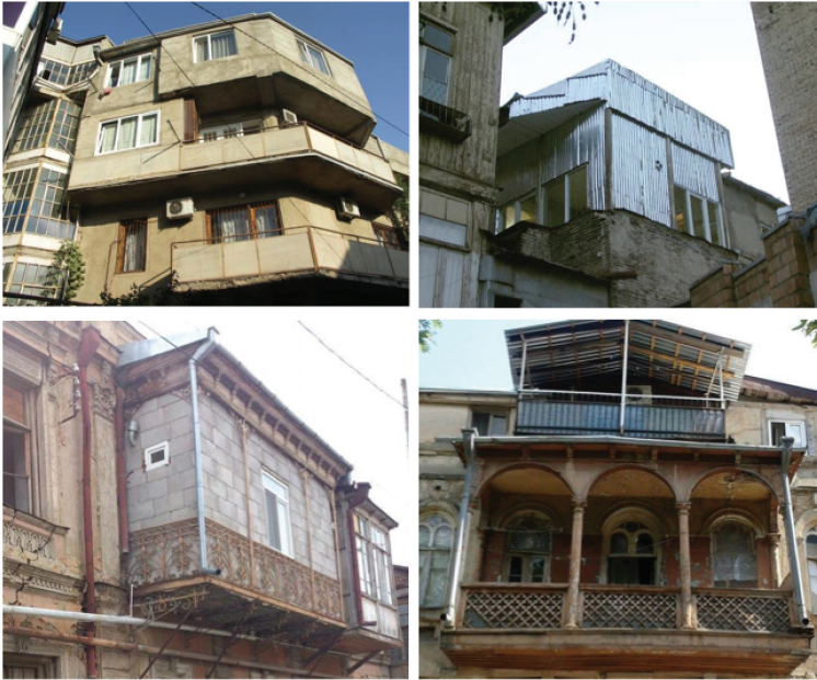
Figure 3. Extensions and additions found on buildings in Old Tbilisi. Additions often accelerate structural damage to old buildings never intended to carry the weight of new floors or materials. © Angela Wheeler.
